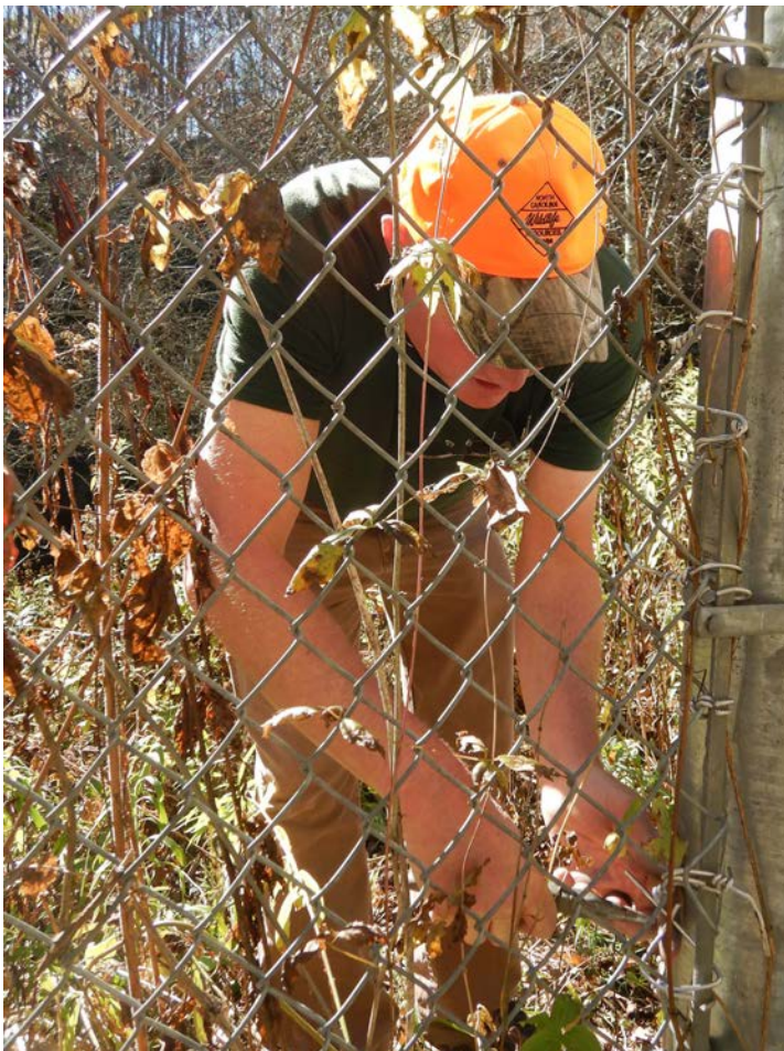
Western Wildlife Diversity Supervisor, Kendrick Weeks, repairs the security fence surrounding an Avery County mine. (Katherine Etchison)
